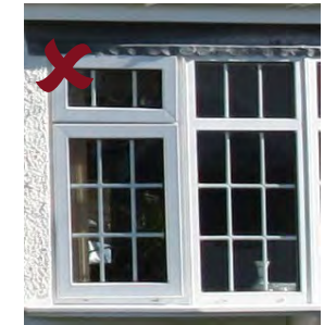
Above: uPVC opening and fixed casement window with overly wide frames
