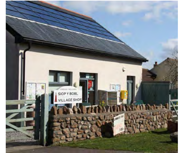
Above: PV installation Llanmadoc
