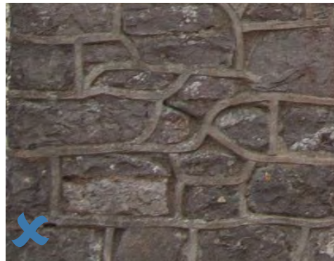
Inappropriate pointing to stone wall
