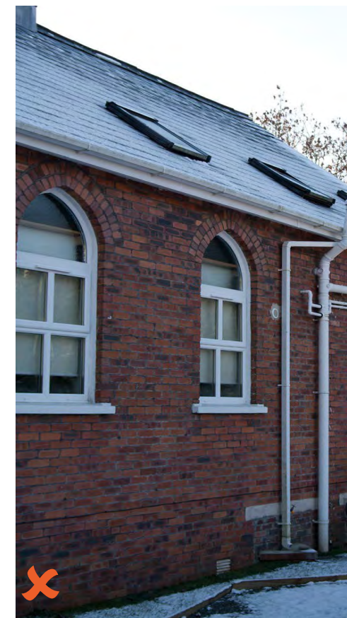
Above: external pipework and timber decking detract from the integrity of this residential chapel conversion
